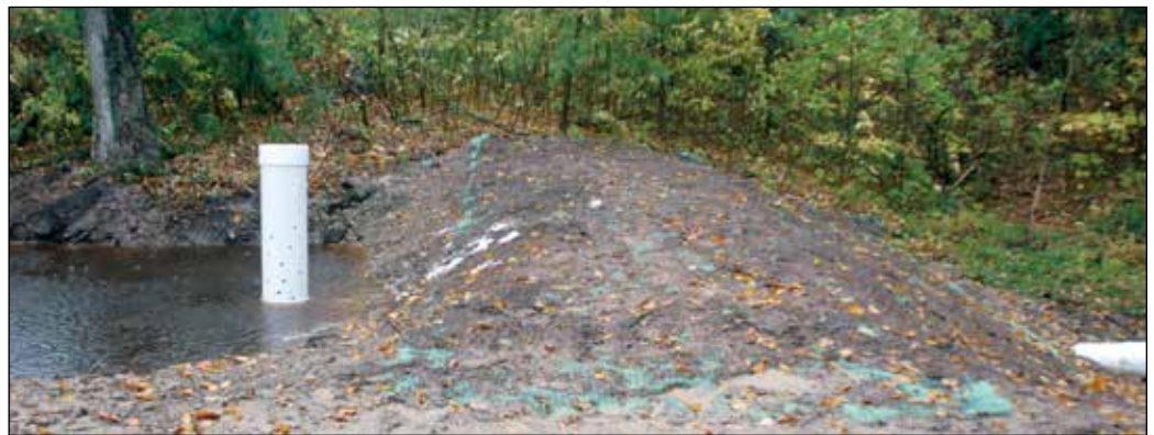
The check dam is a small dam with an overflow pipe connected to a culvert beneath the dam.
